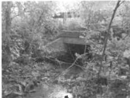
Wilson Avenue Failing Culvert (East Side)
