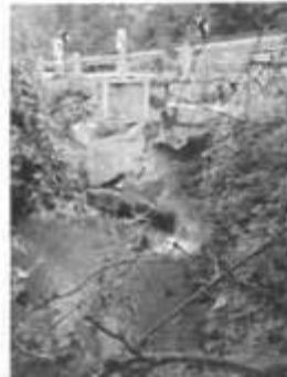
Wilson Avenue Failing Culvert (West Side)
