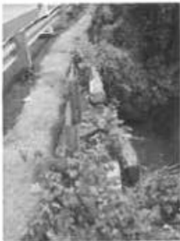
Wilson Avenue Failing Culvert (West Edge of Pavement)
